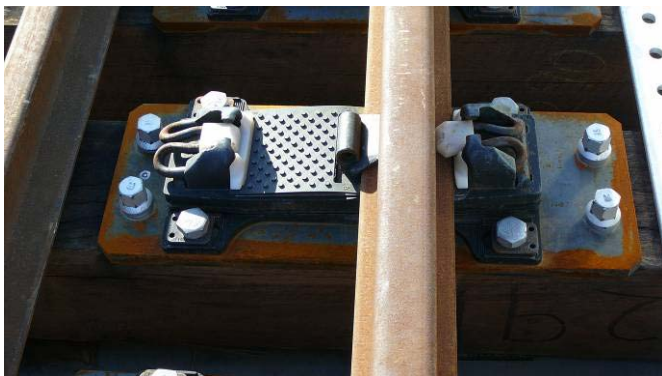
Photo – View of Dual Rail Vipa Fastening System on Lift Up Bridge Span with Std Gauge Rail To Be Installed
