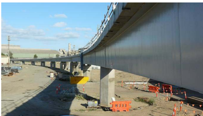
Photo – View of Approach Bridge with Steel Box Girder near and Prestressed Concrete Girders in Distance
