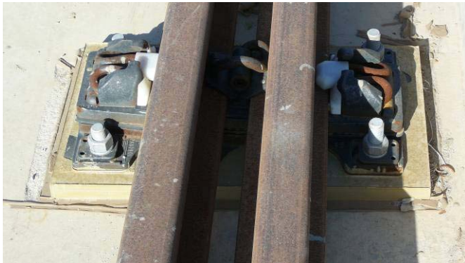
Photo – View of Dual Rail Vipa Fastening System on Fixed Bridge Span
