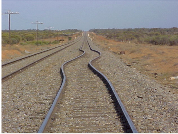
Figure 4 – Typical track buckle
