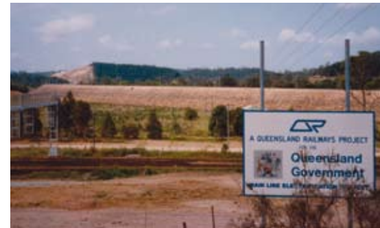
The Eumundi deviation under construction as part of MLE. A plaque nearby unveiled on 21 January 1989 notes that it “...permits the operation of larger and faster trains.” Photo: Philip Laird
