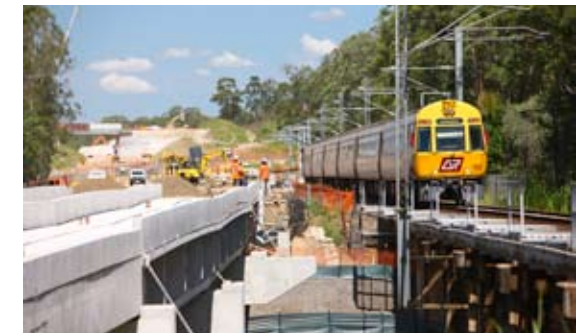
A QR electric train negotiates the single track between Caboolture and Beerburrum. This track is currently being duplicated on an improved alignment. Photo: Trackstar Alliance
