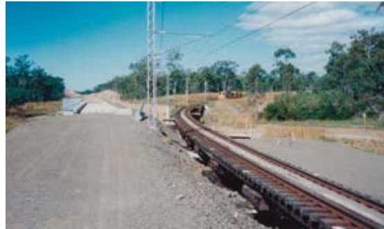
The 12.5 km Watalgan deviation under construction in May 1995 as part of MLU. As noted by a 1996 QR Facts Sheet this project allowed "... trailing loads to be significantly increased."
