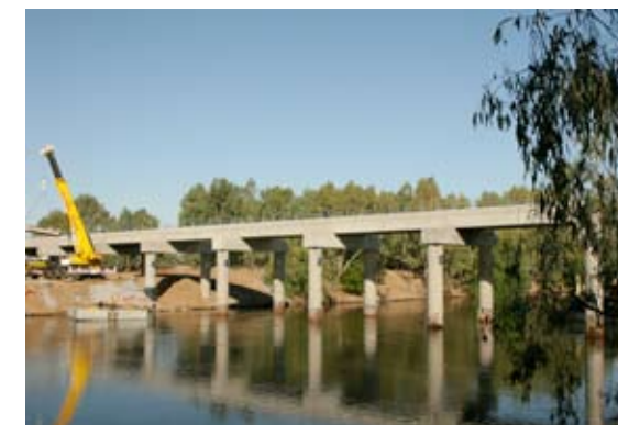
New rail bridge at Wagga Wagga. This bridge over the Murrumbidgee River was constructed in record time by the ARTC and commissioned in January 2007. It replaced a 1880 structure with a long standing 20 km/h speed restriction. Photo: Mark Carter
